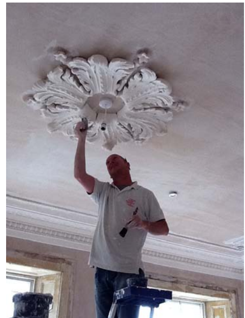
Reconstruction of ceiling rose to original design
